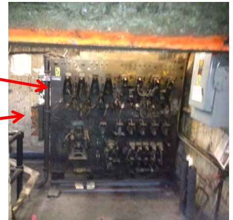
Arch flash concern?
